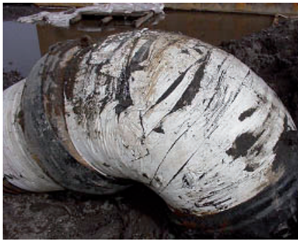
The polyethylene tape has wrinkled and split
