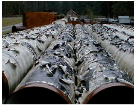
In other areas the polyethylene tape has flaked and peeled
