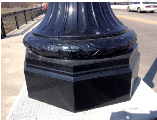
After two years Plascoat PPA 571 on this column looked as good as new.
