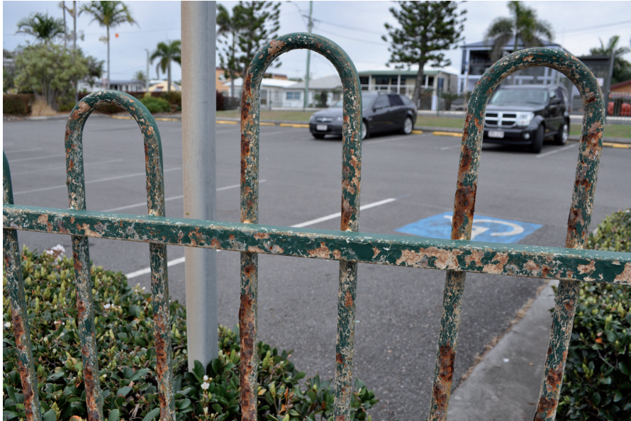
In 1996, after six months of been exposed to sea salt in the air, the polyester coating had failed. The fence was then recoated with Plascoat PPA 571.
