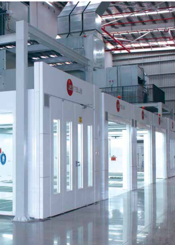
Above: Spray booths in Axalta's NSW Training Centre are fitted with a heat recovery system.
